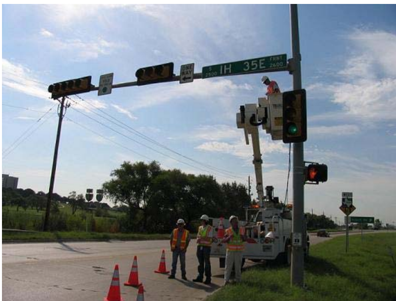
Figure 6.2.3 Mast Arm 2 at the Southwest Corner of the South Intersection of I-35E and Bonnie Brae St. in Denton, TX
