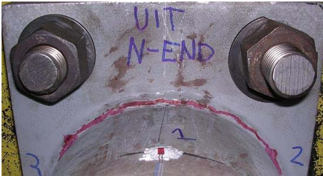
Figure 8.3.2 Highlighted Fatigue Crack on Specimen DU Mast Arm Weld Toe Along the UIT Application Line (90,680 cycles)
