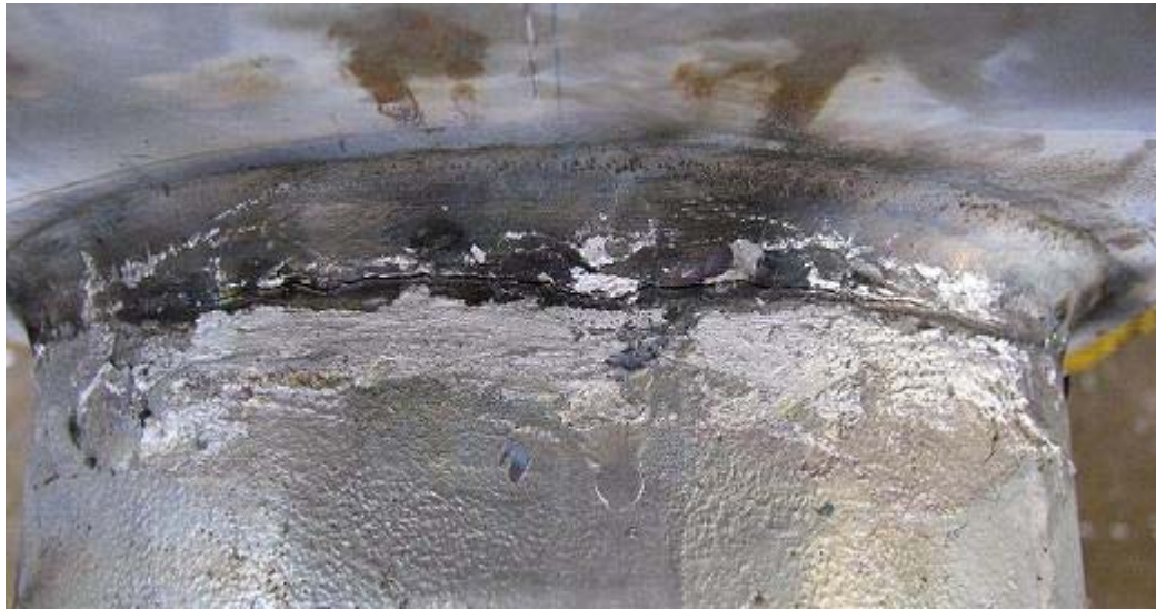
Figure 4.4.5 Mast Arm TXuCLGP After 3 rd Controller-Reported Failure (117,461 cycles) and After Removal of All the Thick Galvanization Repair
