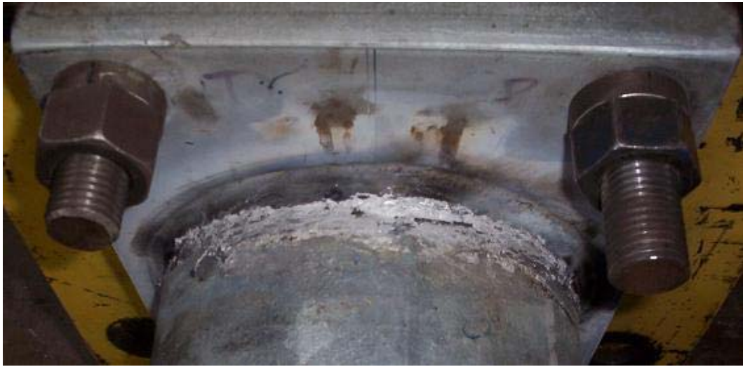
Figure 4.4.4 Mast Arm TXuCLGP After 2 nd Controller-Reported Failure (109,411 cycles)
