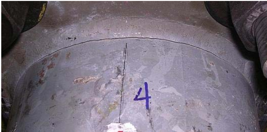
Figure 8.3.5 Close-up of Fatigue Crack Along Mast Arm Weld Toe of Specimen DN (224,905 cycles)
