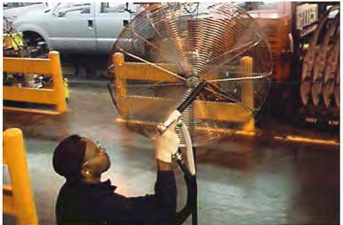
Manfan in an automotive assembly plant being cleaned in-place with dry ice blasting.
