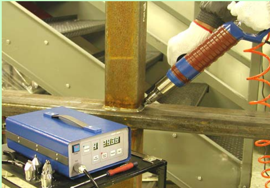
Use of basic UP system for fatigue life improvement of tubular welded joint
