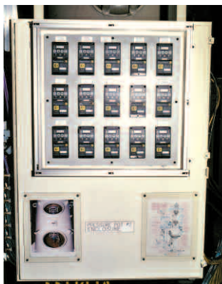
Pressure vessel control panel.
