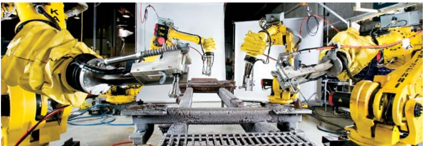
Figure 1. Robotic waterjet cleaning cell installed at a United States-based automotive facility.
