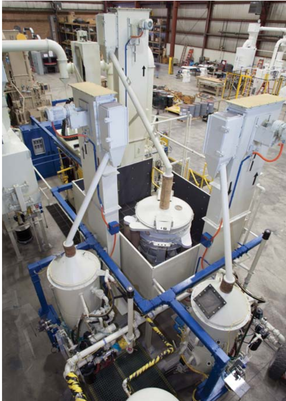
Looking down at the two pressure pots, the two elevators and the Sweco separator. The Sweco is housed in a foam-padded enclosure to reduce noise. Each pressure vessel has two MagnaValve media valves and the Sweco screens 100 percent of the media with a five-deck screening system.
