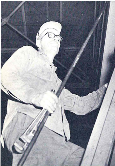
Plumber Bob Simper climbs to the rafters to install a new pipe.
